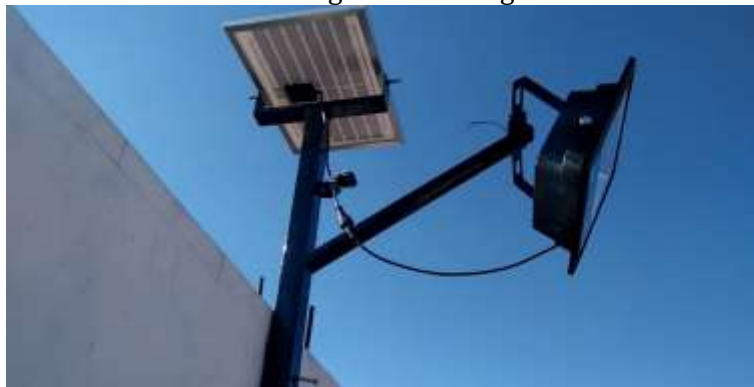
Figure 4. One of the positions for installing solar chell lights at the Panti location
